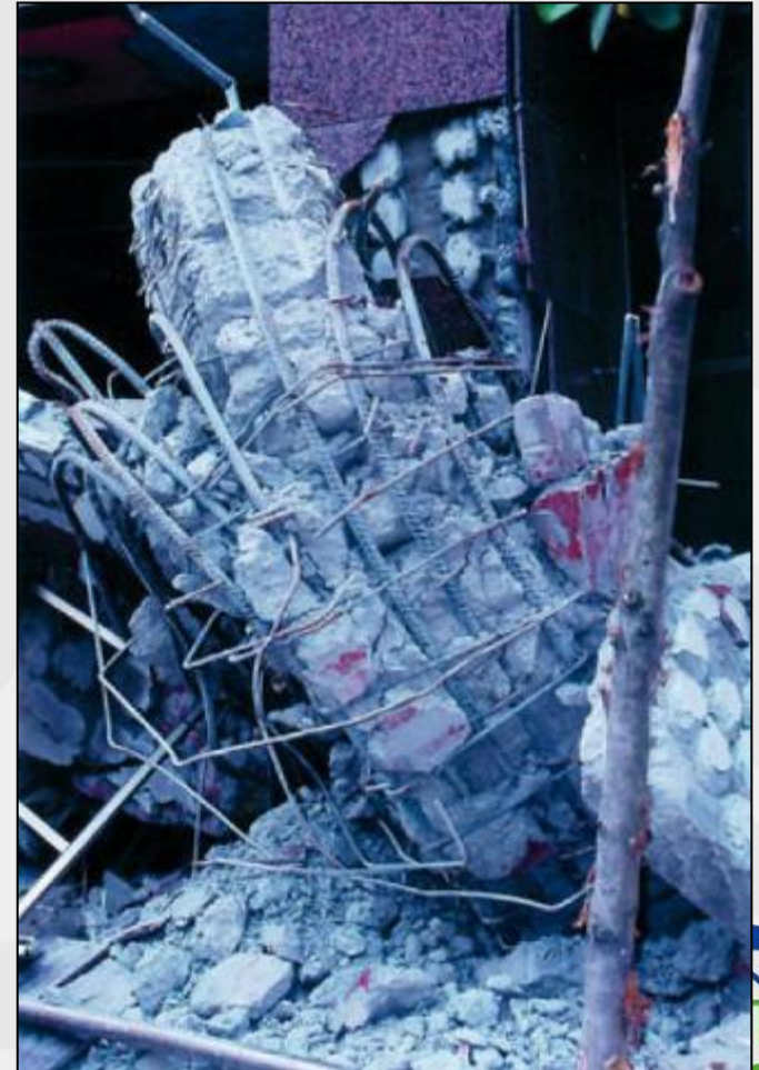
柱斷裂，樓房崩塌
