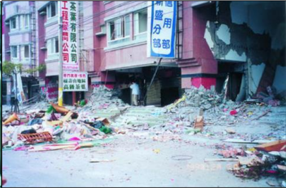
柱斷裂，樓房崩塌
