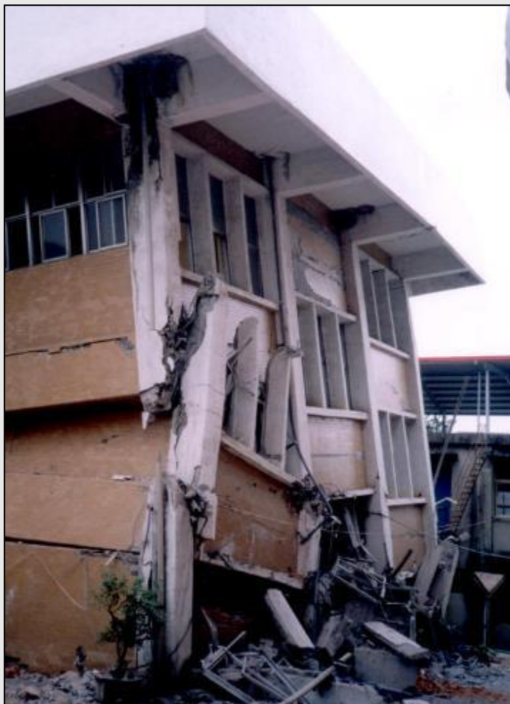
柱斷裂，樓房崩塌
